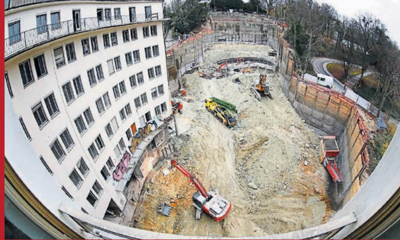
Through the fish eye lens: The major construction site at the Kureck where there is some progress at last. Luxury apartments, office and flex space are planned here. The high-rise block will be demolished next year. A residential tower will be erected.
